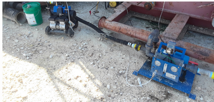
The 50 XTB nanobubble generator treated produced water in a third tank.
