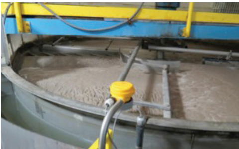
Dissolved Air Flotation tank at Hershey Creamery being skimmed after the Nanobubble Generator installation.
