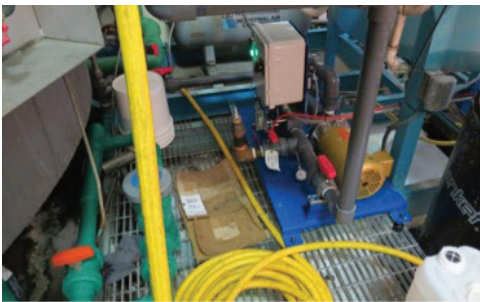
Moleaer Nanobubble Generator installed at Hershey Creamery.
